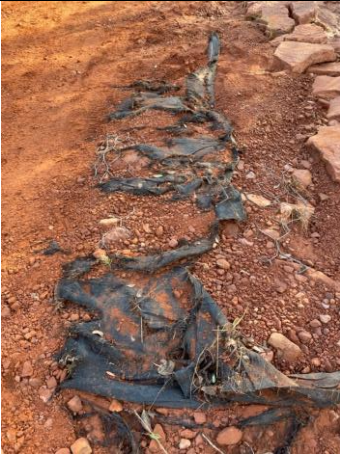
Exposed gabions (metal mesh rock-filled cages used to support trails) on Bell Rock Pathway
